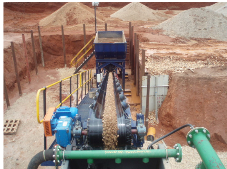
Feeding of the DMS plant
